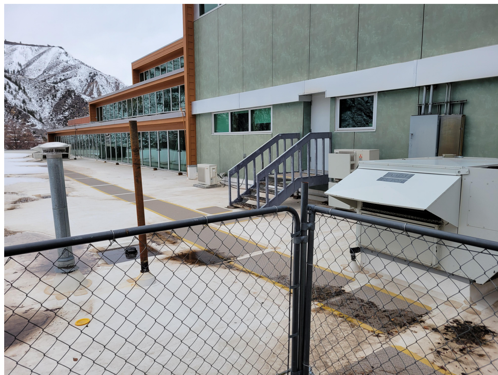
EXISTING ROOF CONDITION ABOVE MINI COLLEGE. SEE DRAWING FOR PHOTO LOCATION REFERENCE
